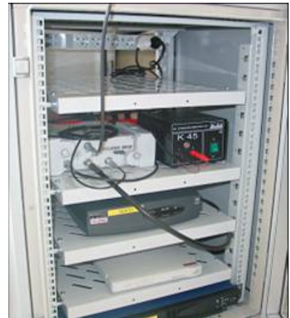
The inside of a FLEPOS station.
