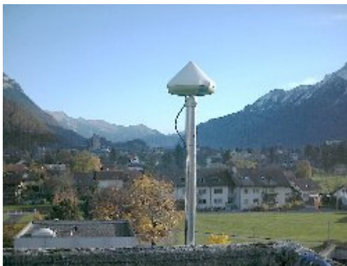
The SWISSAT station in Interlaken
